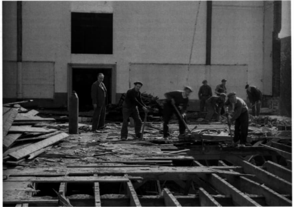
Fig 6: Gallery 29 (formerly Agricultural Implements) in course of demolition, 22 April 1949, looking east. Close examination of a scan of this photograph at extreme brightness reveals the horn still in existence in the dark area just beyond the gallery entrance.
