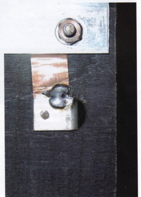
close-up of soldered copper straps
