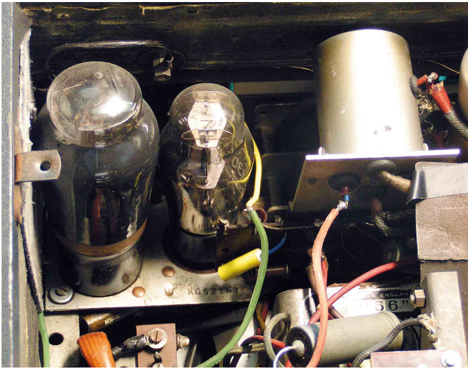
Output valve and rectifier
