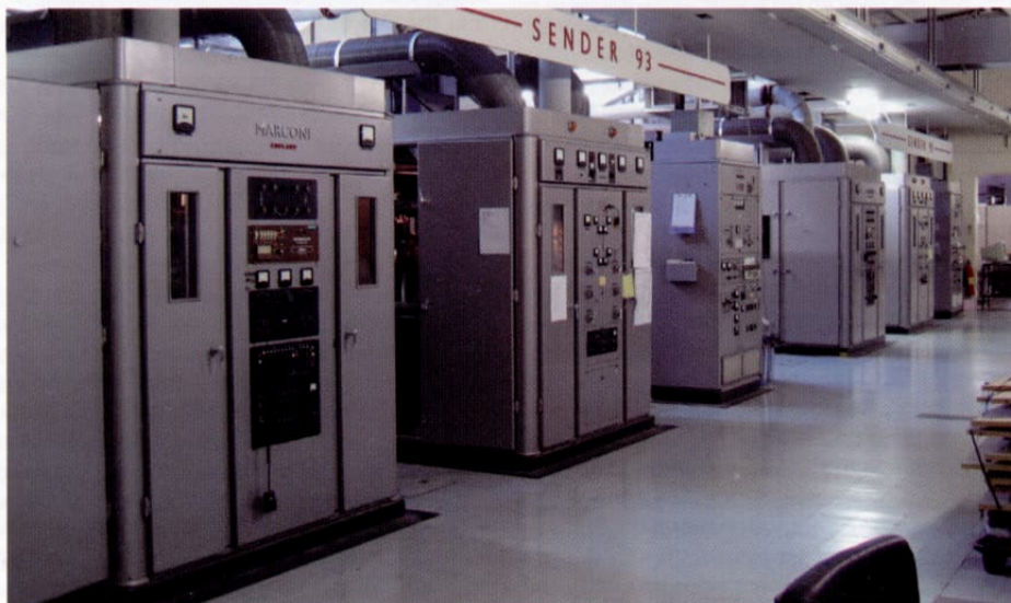
Main transmitter hall with 1960's Marconi transmitters
