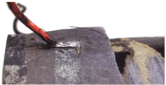
The corroded field wire
