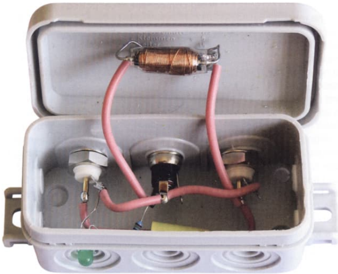
Inside the power feed box
