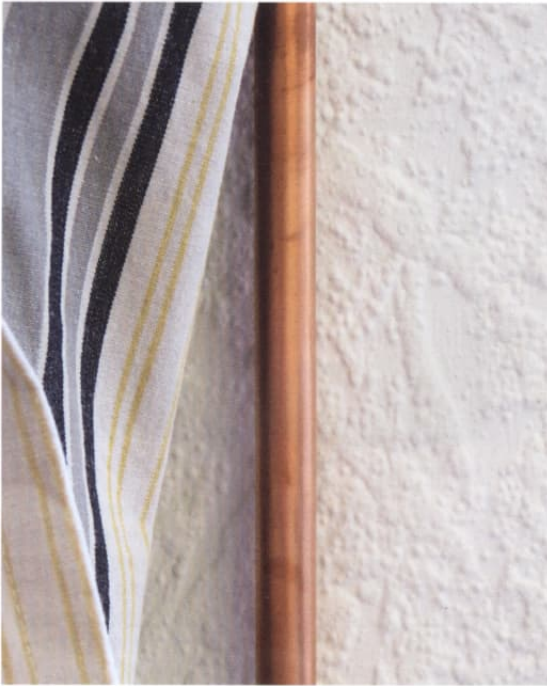
Big loop vertical runs behind the curtains
