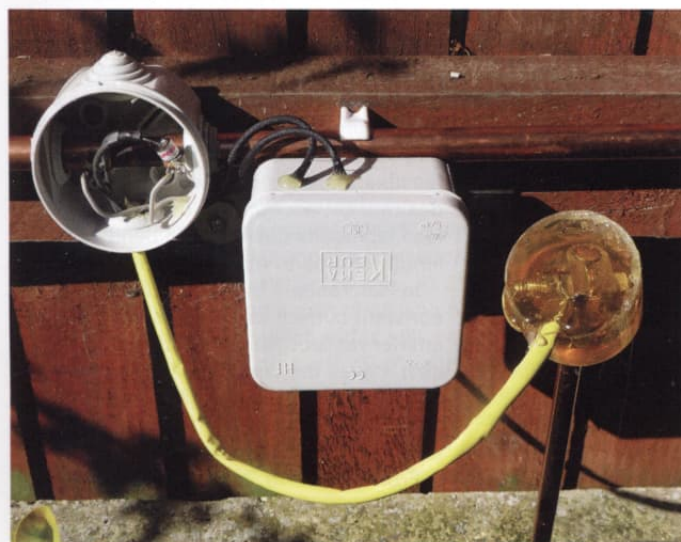
The loop connections and Earth stake
