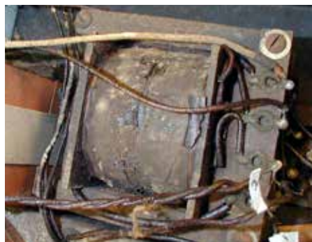
Fig. 16 – Transformer before with its grimy perished insulation.
