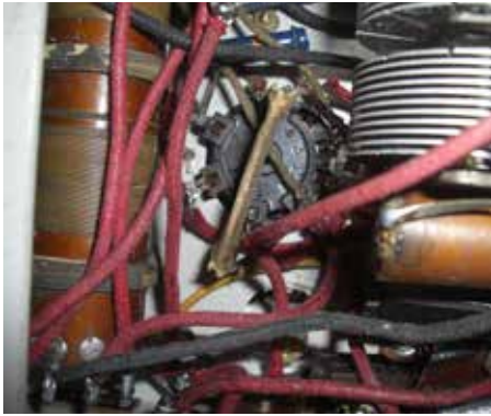
9. Close up of the rubber cloth covered wire
