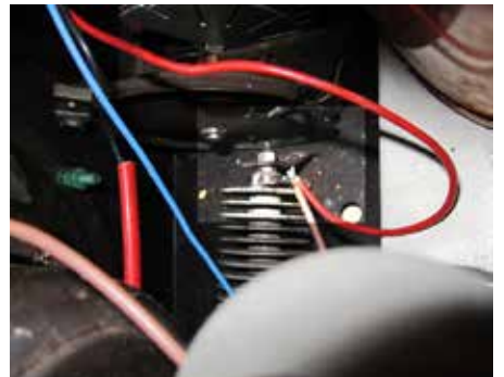
Fig. 13 – Richard's rectifier placement photo
