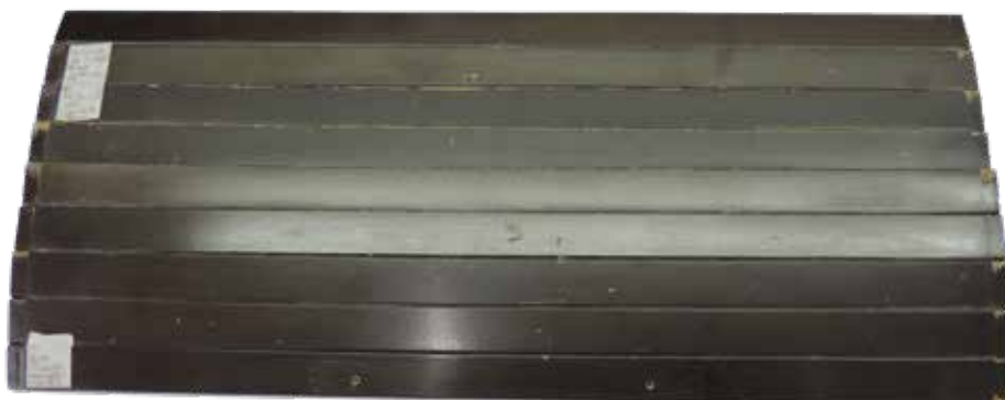
The roll top timber slats in the process of being assessed for colour matching due to the poor and faded condition of the existing finish.
