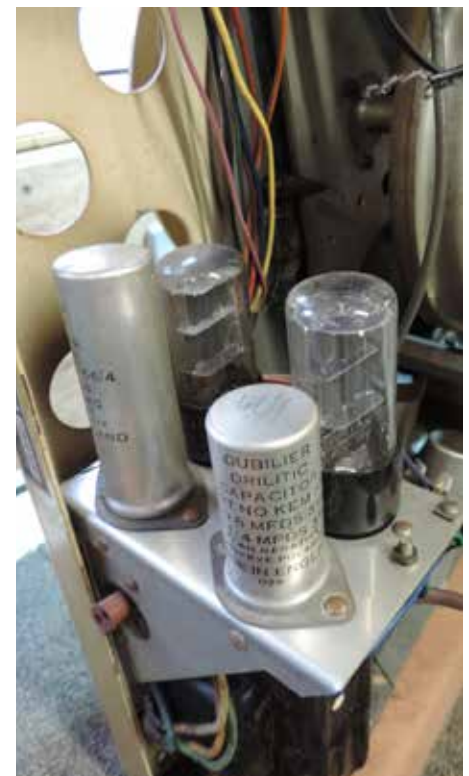
The power supply unit as found. The two 6X5G rectifiers and associated smoothing can be seen here.
